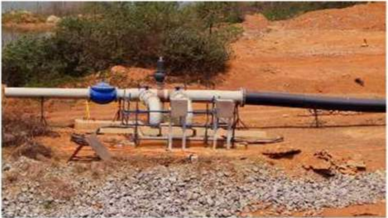
INSTALLATION OF RAW WATER PUMPS AND HEADER PIPES FOR NEWMONT GOLD CORP AHAFO MINE
