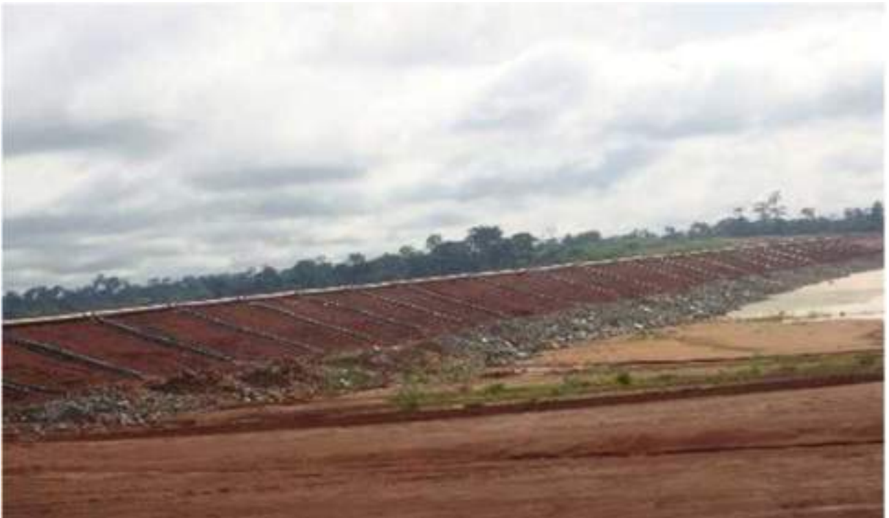
INSTALLATION OF 630 TSF PIPELINE AND SPIGOT DROPPERS FOR NEWMONT GOLD CORP AHAFO MINE.
