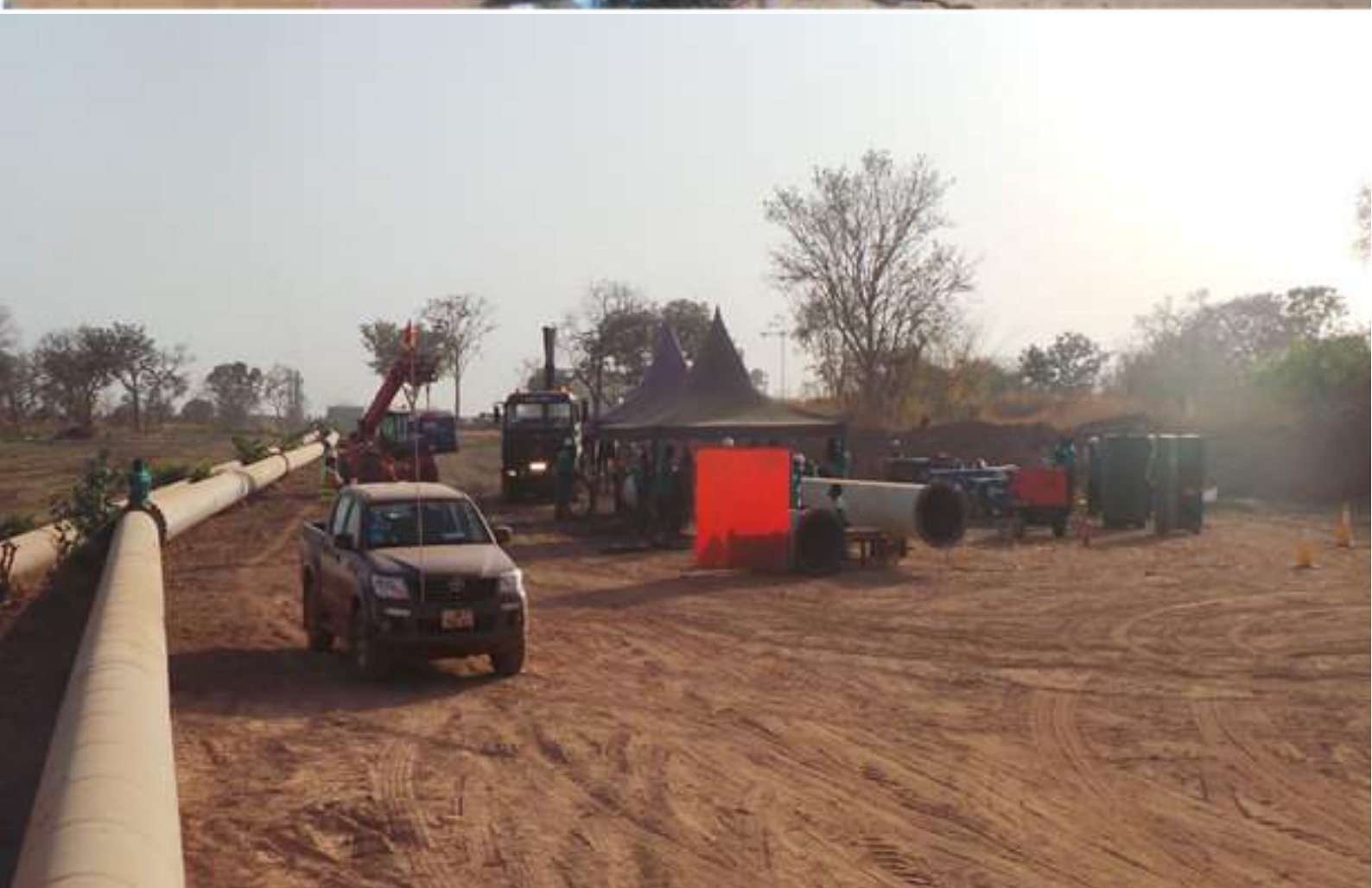
INSTALLATION OF 8KM 800mm STEEL PIPES FOR ANGLOGOLD ASHANTI TSF SAG SIGUIRI
